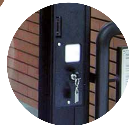
FLOOR CONTROL PANEL
